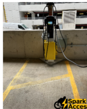
Clear Ground space as part of an access aisle; ChargePoint in Ann Arbor, MI, using sheathing instead of bollards for unobstructed reach.
