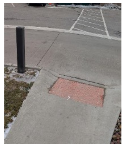
Accessible route example, using the existing route from the entrance to the trash collection location
