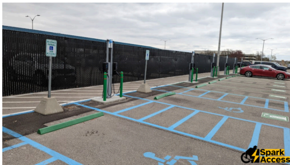
Example of Accessible L2 charging at a Flo installation
