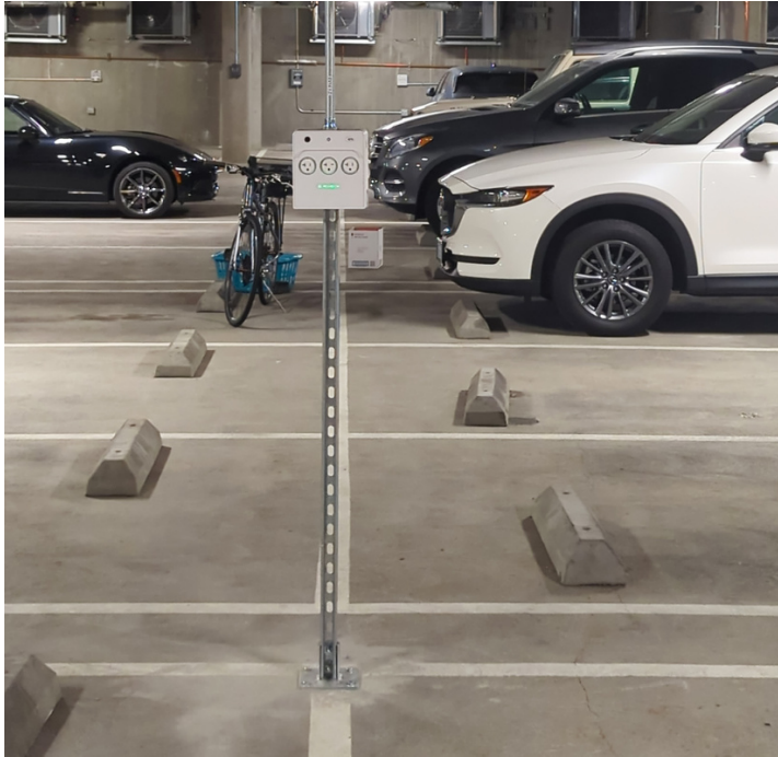
GoPowerEV SmartOutlets in the University Terrace Garage
