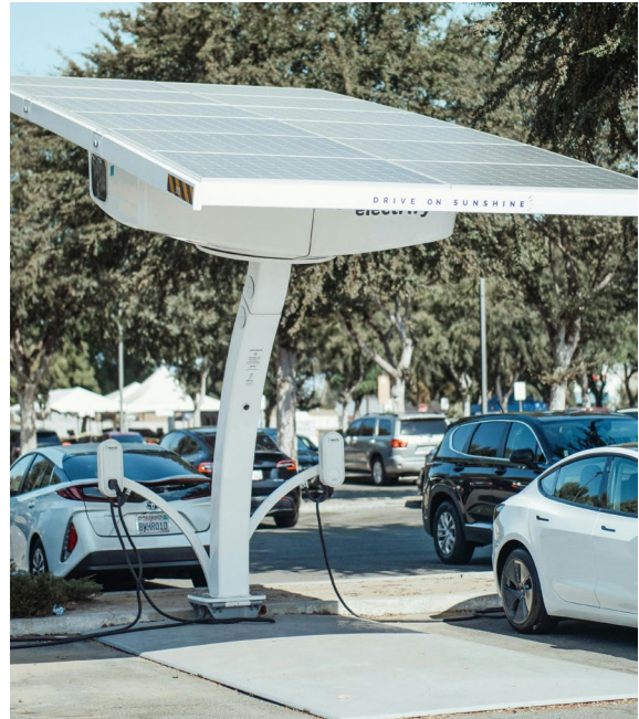
DEDICATED EV CHARGING
